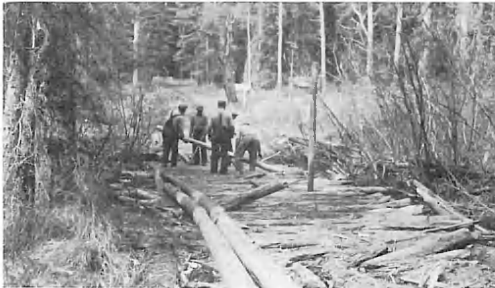
Settlers repairing roads and bridges between Ta- kysie Lake and the settle- ment.
