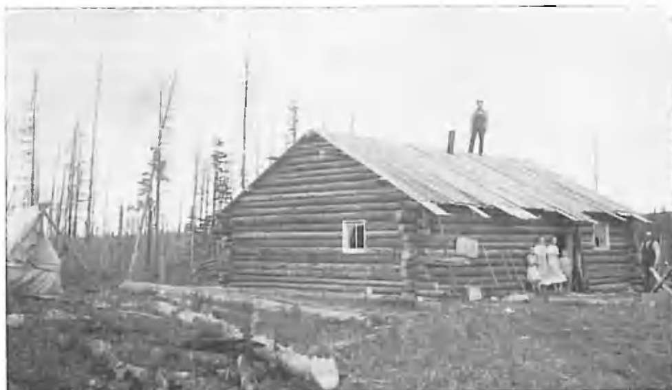
Cheslatta, B.C. July 25th, 1940. J. Petkau's house under construction. Settler and family standing near door.
