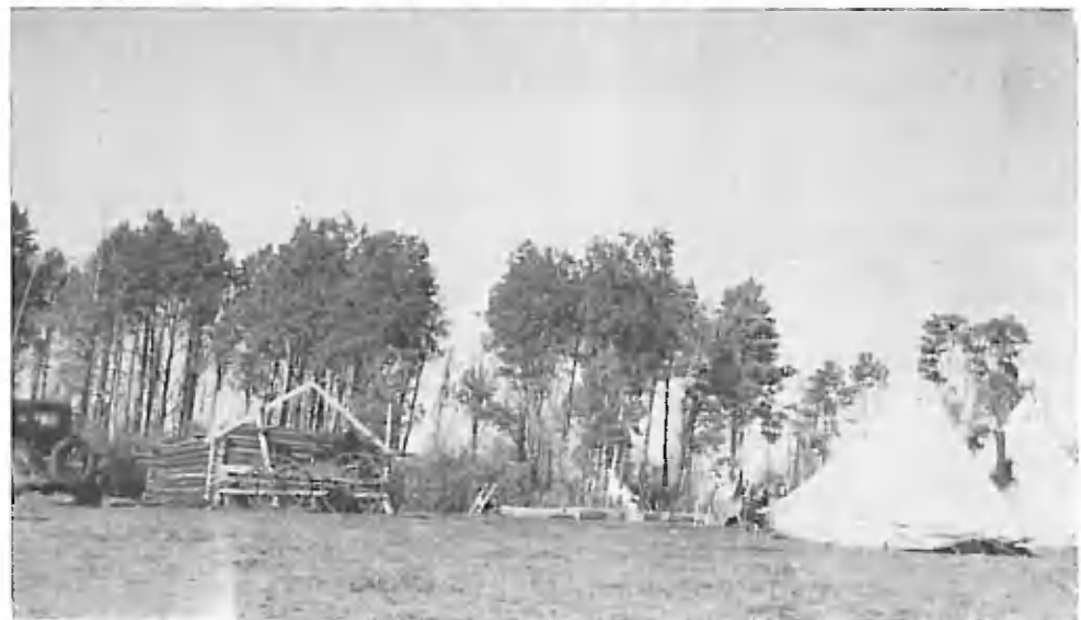
House under construction. Temporary quarters of H. K. Bergen at Cheslatta, B.C.
