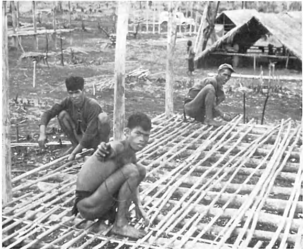
In the background is the roof which was built first under which refugees are living until the rest of the house is completed.
