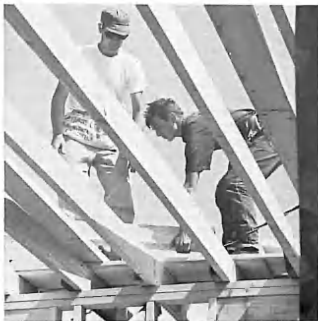
M.D.S. workers from Lancaster County erect home in Dunlap, Indiana, following tornado, 1965.
