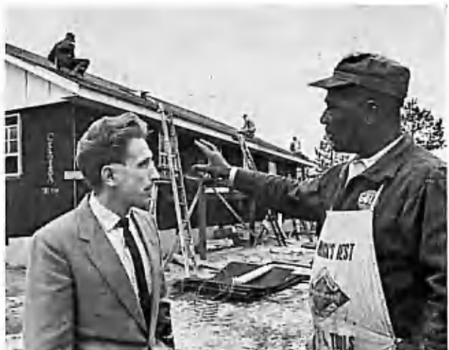
M.D.S. helps rebuild Pleasant Grove Baptist Church, Mississippi, one of the thirteen churches the organization is helping rebuild after they were bombed or burned.
