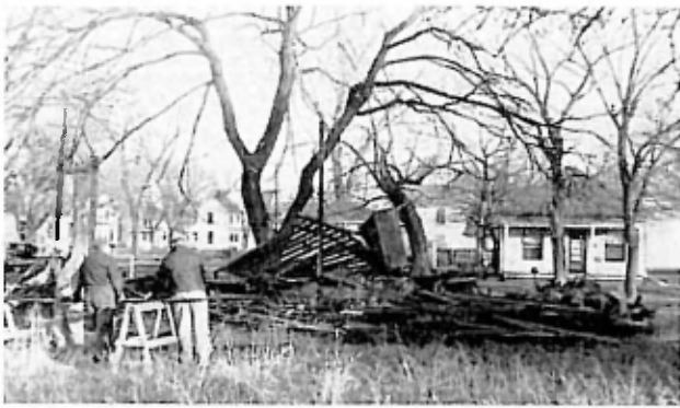
Rebuilding a house in Topeka, typical of work of Mennonite men in storm and flood areas of Nebraska, Kansas, Oklahoma and Arkansas.
