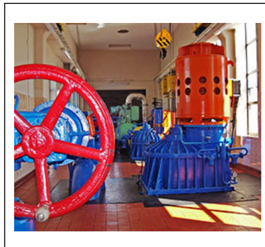
Pumping Station in the Werder Photo: Robert Friesen
