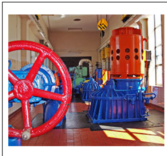
Pumping Station in the Werder
